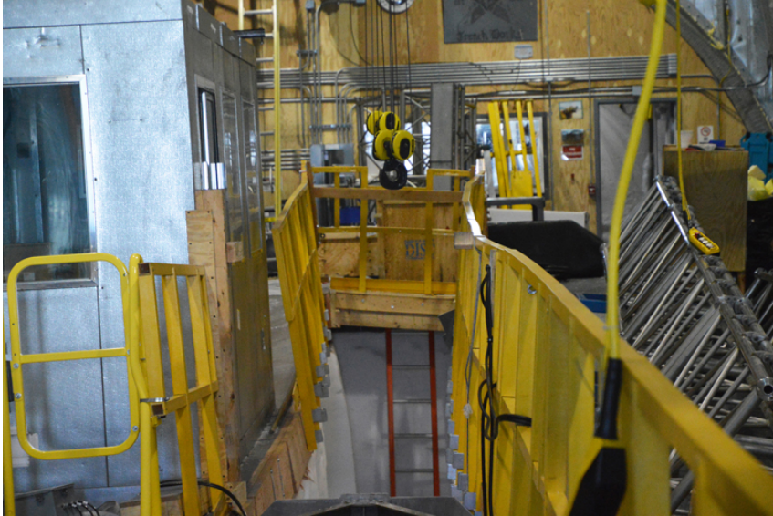
View of the inside of the drilling side of the arch showing the buckling of the railings due to the uneven buckling/deformation of the floor. Photo: Don Voigt.
