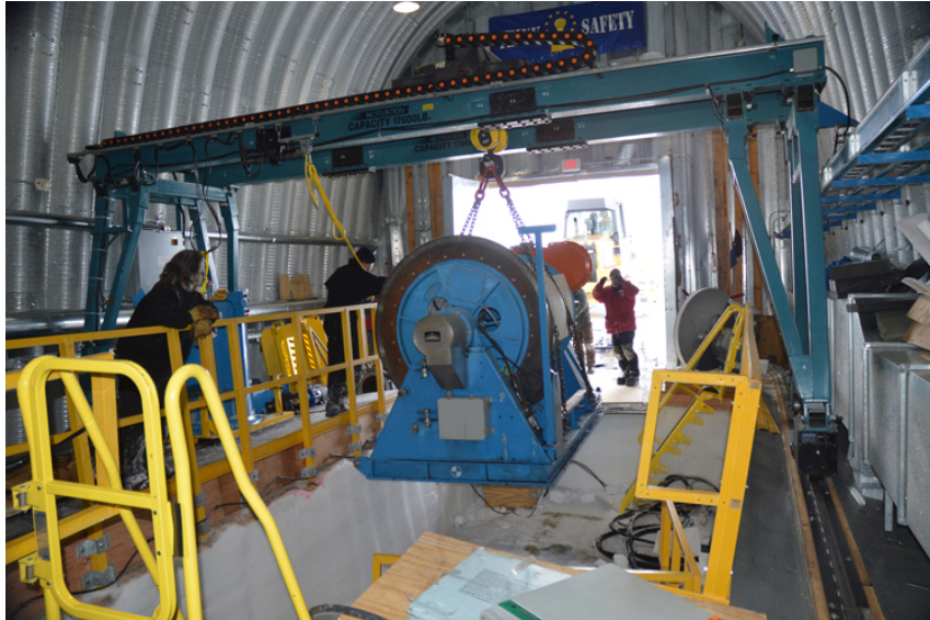
Lifting the DISC Drill's winch drum out of the winch pit. Photo: Don Voigt.
