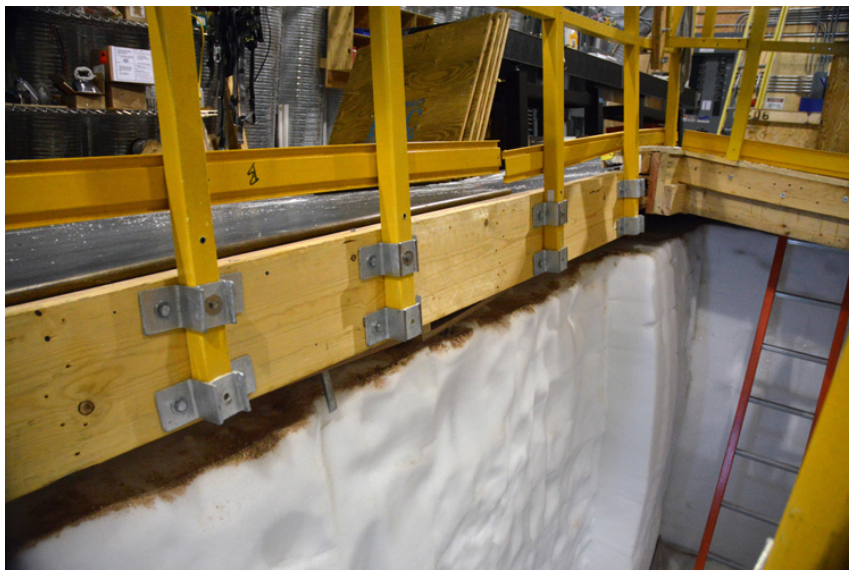
View of the inside of the drilling arch showing the uneven deformation/buckling of the floor. Photo: Don Voigt.
